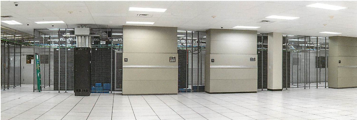
20,000 SF hardened Data Center
