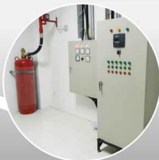
Fire Extinguishing Devices
